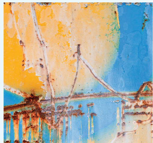
Painted by rust
