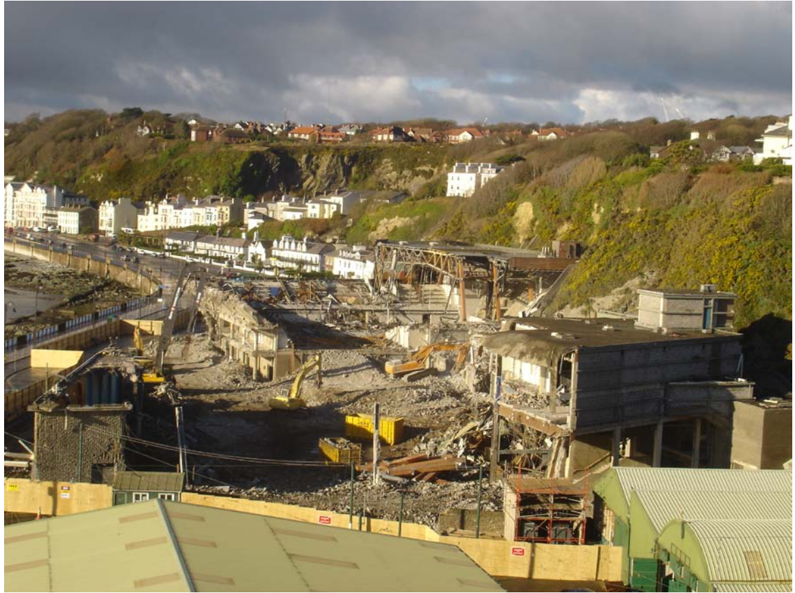
Figure 9.5: The demolition nears completion. The only parts of Summerland left remaining in this photograph are the NE corner of the Piazza floor and part of the concrete wall fronting King Edward Road. (Photograph: Ricky Rooney and James Turpin)
