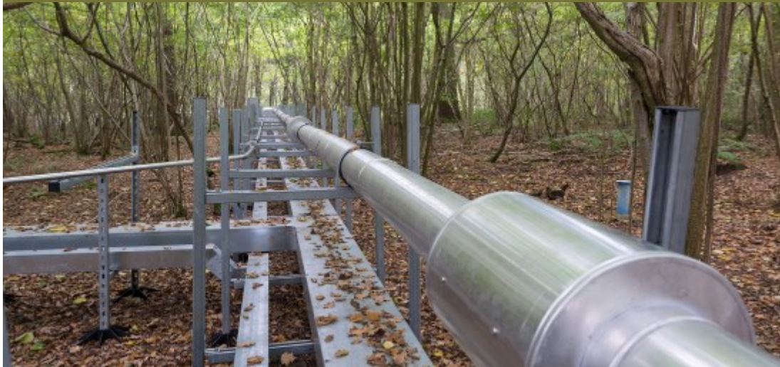
Approximately 1,000 metres of pipework carries carbon dioxide (CO 2 ) throughout the woodland Photo credit, Andrew Priest Photography www.prophotographers.co.uk
