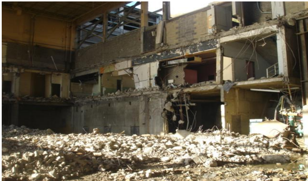
Figure 9.4: The demolition of Summerland. This photograph was taken in the Sports Hall. The remains of the Carousel staircase that descends from the Piazza floor to the Derby Bar can be seen on the right-hand side of the photograph (Photographs: Ricky Rooney and James Turpin)
