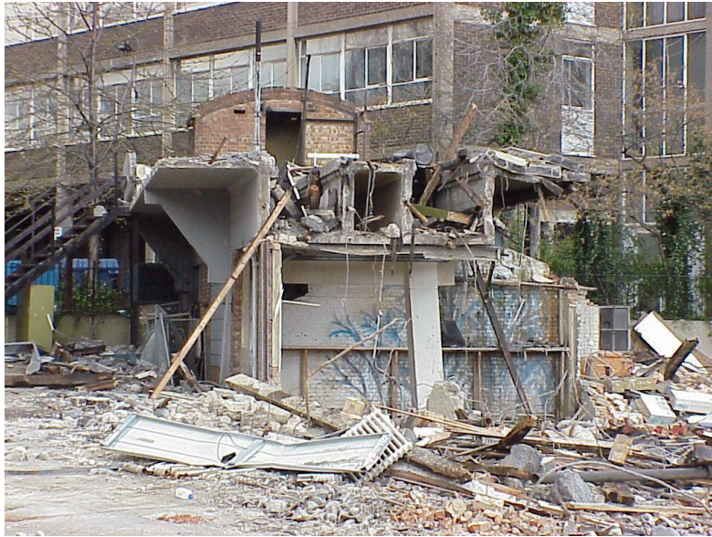
16 April, 2001 – demolition of the last concrete track section and A-frame supports, North End Road, near Wembley Park Underground station
