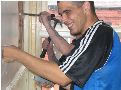
Latch Project, Leeds: A trainee working on an empty property being brought back into use (reproduced with permission of self-help-housing.org)
